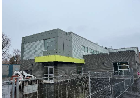
Exterior photo of the north elevation of the new childcare/classroom addition showing completed brick, metal panels, metal siding and windows.
