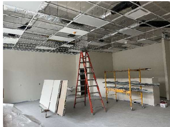
Interior photo looking to the northwest of new kindergarten room currently under construction ready for above ceiling inspections.
