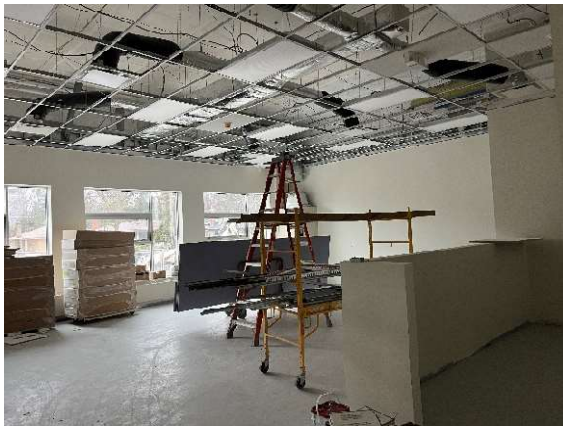
Interior photo looking to the southwest of new kindergarten room currently under construction ready for above ceiling inspections.
