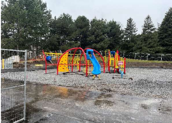
Exterior photo looking to the southwest of the recently installed play structure ready for soft scaping works.
