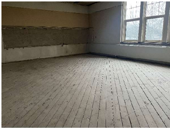
Interior photo looking southeast of existing classroom showing demolition works completed and ready for new subfloor installation.
