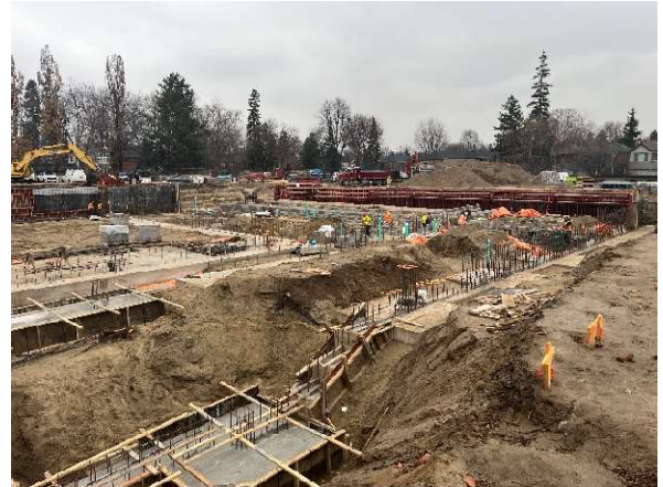
Exterior photo looking to the northeast showing foundation progress of the new addition.
