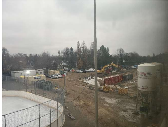
Exterior photo looking northeast from third floor classroom showing site trailer and forming foundation wall progress of future 3 storey addition.
