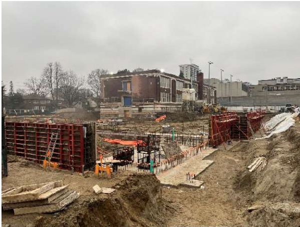
Exterior photo looking southwest at the east elevation of the 1920's building showing foundation progress.
