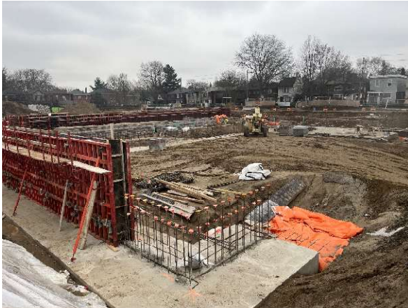
Exterior photo looking to the southeast showing foundation progress of the new addition.
