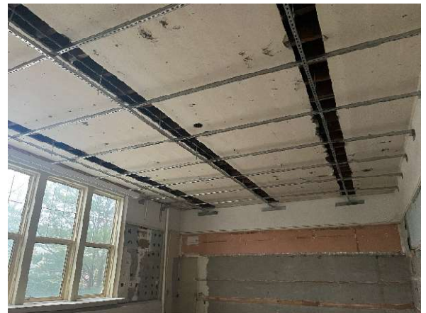
Interior photo completed Unistrut suspension system in existing classroom currently under renovation.
