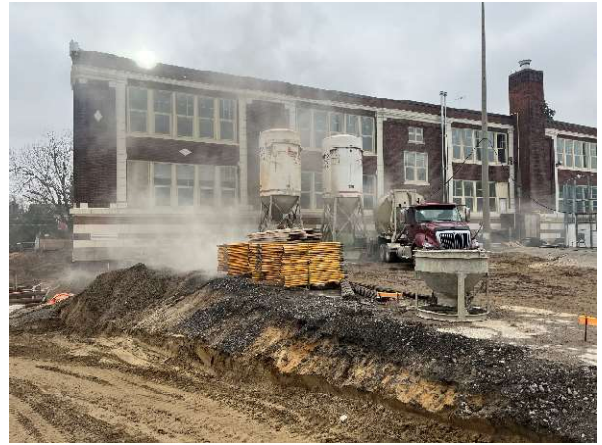
Exterior photo looking south showing the mortar silos used for masonry construction.
