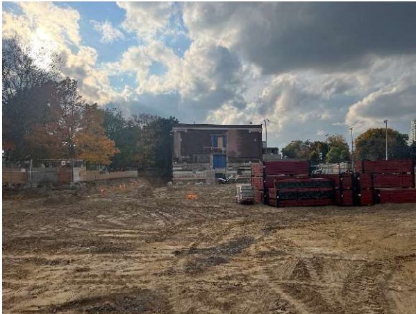
Exterior photo of the east elevation showing the 1960's building completely demolished and exposing the interior wall of the 1920's building.
