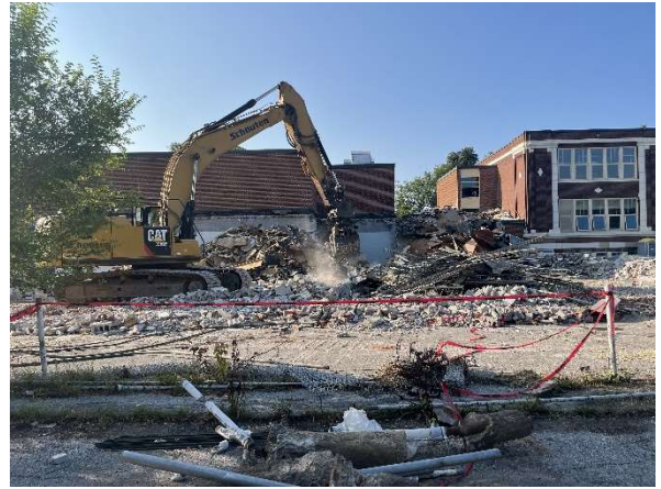
Exterior photo of the north elevation of the 1960s portion of the building currently being demolished.
