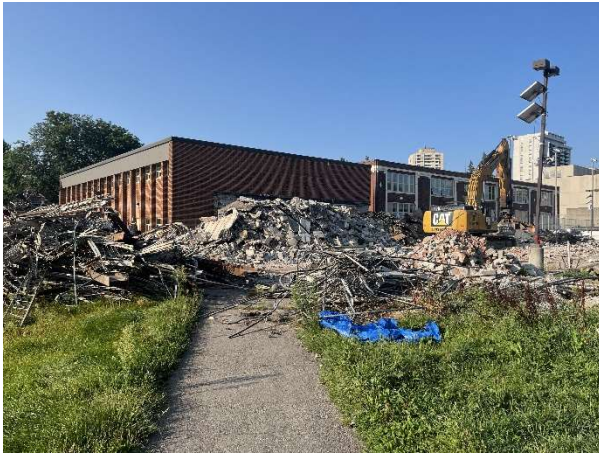
Exterior photo of the northeast elevation of the 1960s portion of the building currently being demolished.
