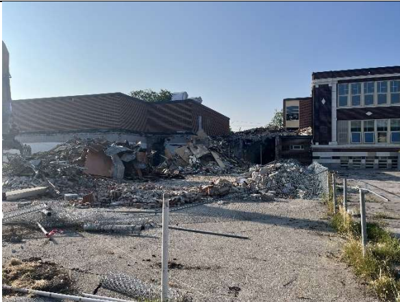
Exterior photo of the northeast elevation of the 1960s portion of the building currently being demolished.
