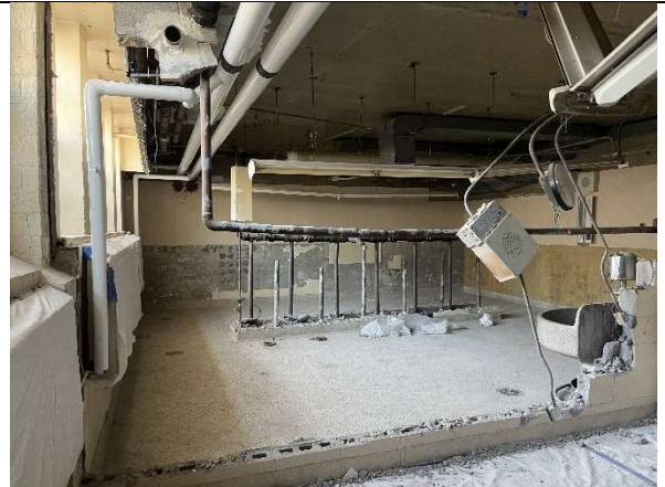
Interior photo of existing ground floor washroom and storage room being demolished and converted into a regular classroom.
